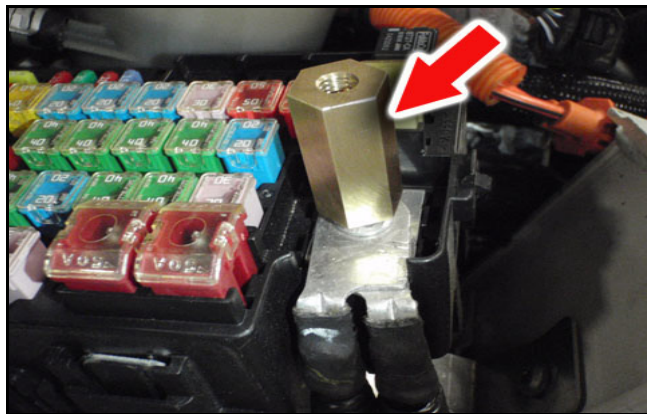
FST9001 - Battery Charging Terminal Adaptor (red arrow) installed on the B+ post in the PDC.
