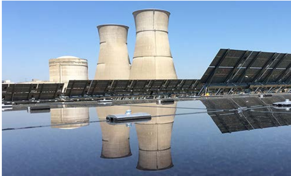
Source: Sacramento Municipal Utility District Rancho Seco Photo https://www.smud.org/en/Corporate/Environmental-Leadership/Power-Sources/Rancho-Seco-Solar-II-Development
